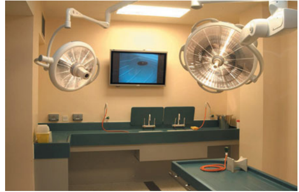
Figure 3.3 Modern forensic autopsy facilities, including directional overhead lighting – with inbuilt video projection and recording capability – to facilitate optimal forensic pathological examinations.
